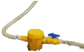
Figure 16: Pressure Relief Valve 34
