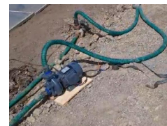
Figure 30: Surface Motor-Pump set 49
